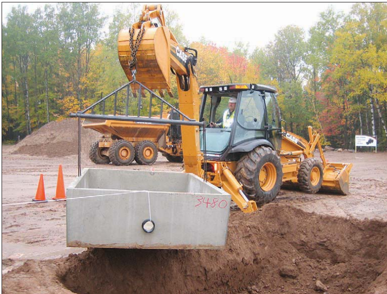
The Case 580 Super N backhoe demonstrates its lifting capabilities at the product review center in Tomabawk, Wis.
